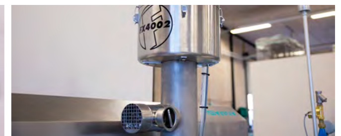
Steam condensation units
