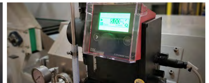
Automatic chemical dosing pumps
