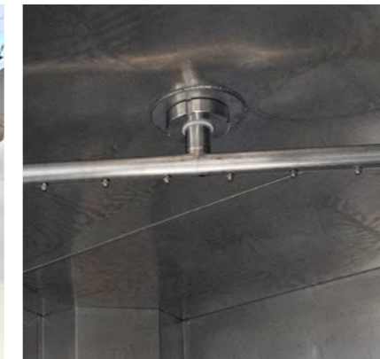
Rotary spray system
