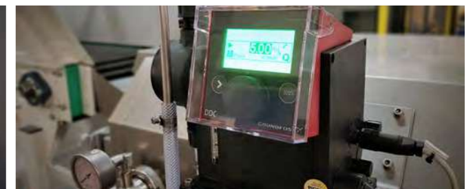
Automatic chemical dosing pumps
